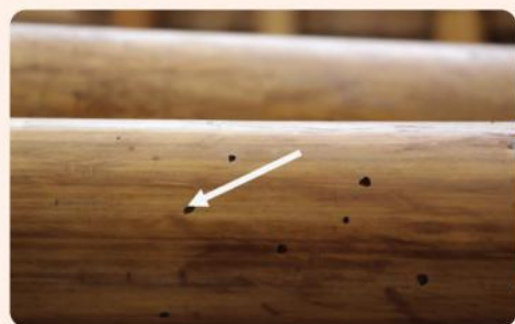
Exit holes on bamboo damaged by beetle
