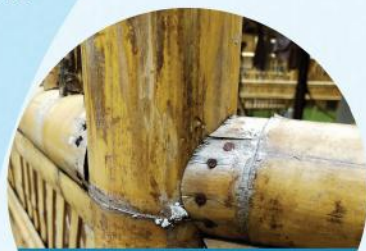
Cracks and splits from use of nails on bamboo jointing
