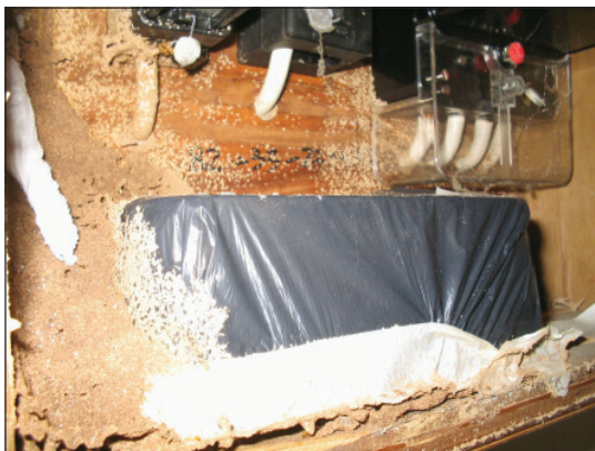
Fig. 6. Switch box infested with C. gestroi .
