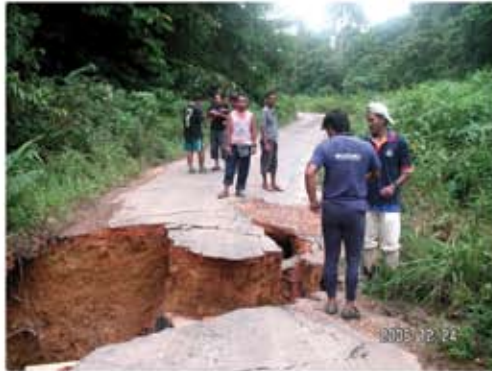
A road that caved in at Peta, Endau-Rompin Johor National Park
